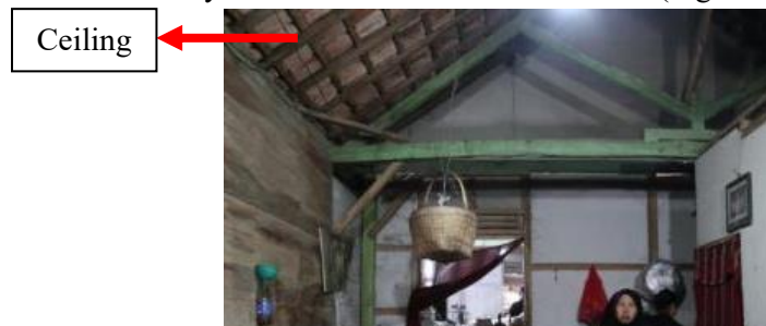
Figure 28. Kitchen Ceiling of Mr. Lasiyo's House Source: Widyaswati, 2023
